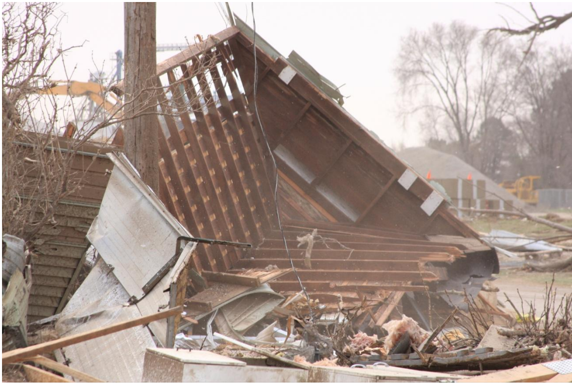
FIGURE 2-3 DAMAGE FROM THE MAPLETON, IOWA TORNADO OF APRIL 10, 2011 SHOWING AN ENTIRE ROOF LIFTED OFF OF ITS SUPPORTING WALLS
